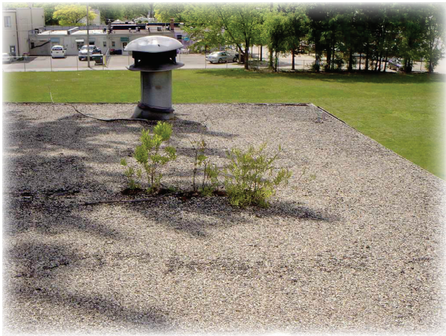
This is not what is meant by a "Green Roof".
